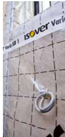
To ensure air tightness continuity, ensure that all penetrations are sealed correctly
